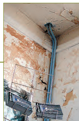
The squat where we live and produce this magazine in is an abandoned building owned by a giant international insurance company. The building was empty for eight years before being squatted in 2000. It's scheduled for major renovations in 2003 because of structural problems such as this leak. Let us just say a few of the clothes got a little wet... (if you're wondering, the company is taking serious action against us in the French courts and we will probably have been expelled from the property by the time you read this).
